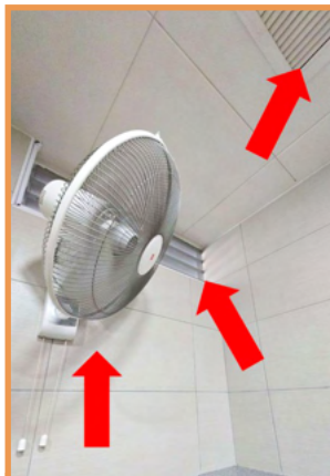
Features to facilitate ventilation (i.e. exhaust fan, louvered window, wall fan)
